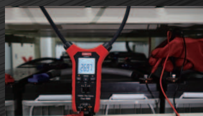
DC current test of Battery modules
