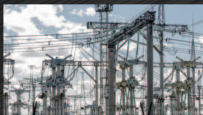
Power distribution station
