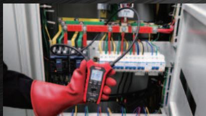
Bus bar current test
